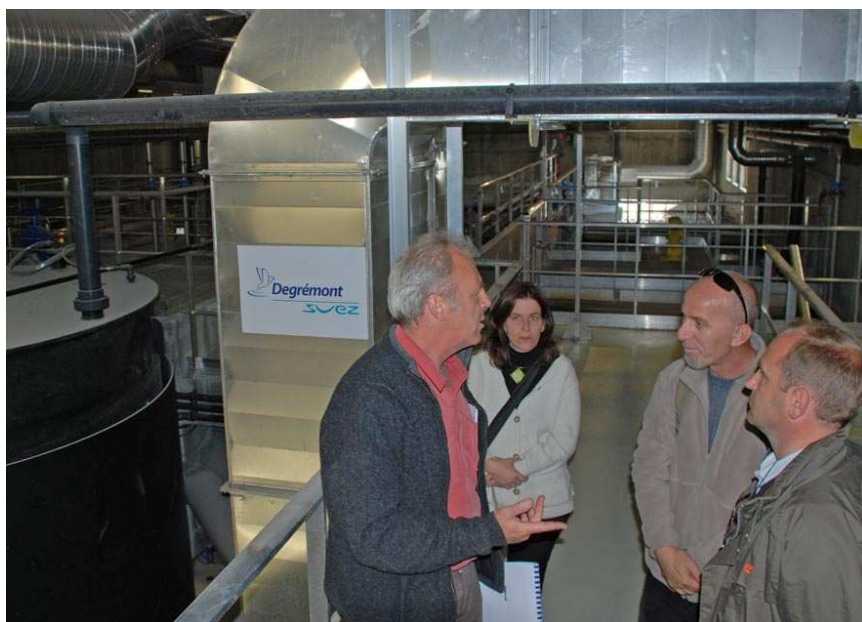
Visit of the Briançon sewage works
